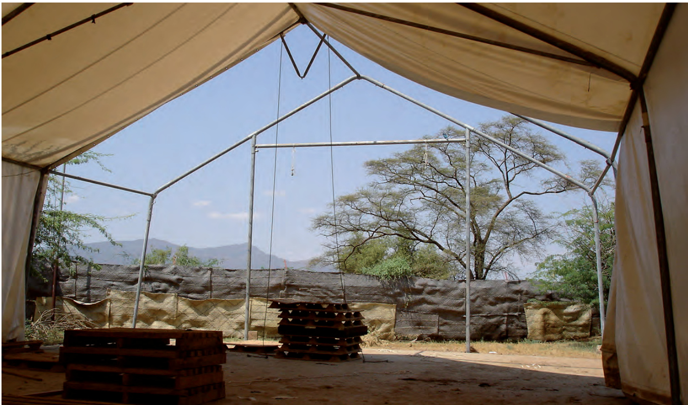
RUB HALL TENT BEING ERRECTED / TENTE RUB HALL EN COURS DE MONTAGE MSF, SUDAN
